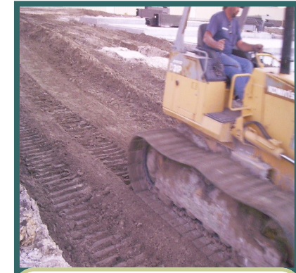
PHOSPHOCRETE™ Looks like typical fill, but cements over time to create a VERY stiff platform on which to build
